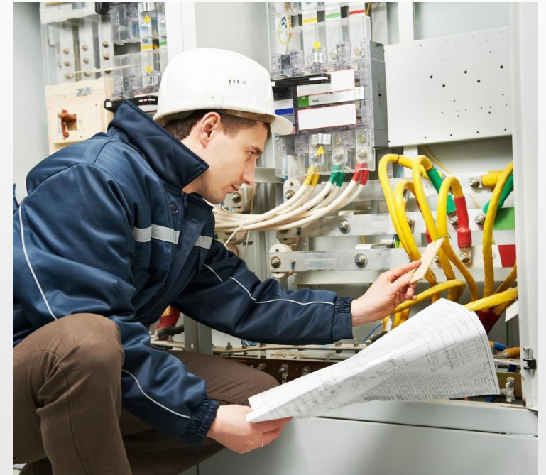
Service and Revamping
